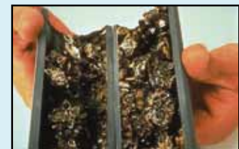
Zebra mussels in a cut-away pipe
